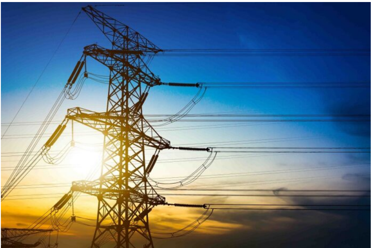
High voltage post or High voltage tower
